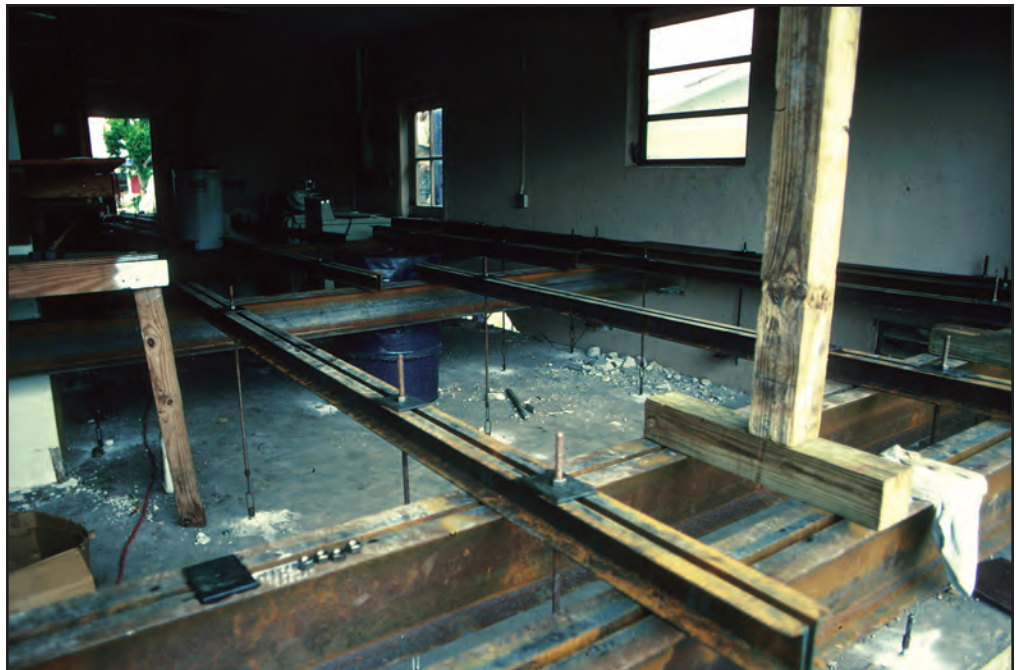
Figure 79 The anchors and hangers connect the slab securely to the beams, enabling the beams to raise the slab along with the rest of the house.
