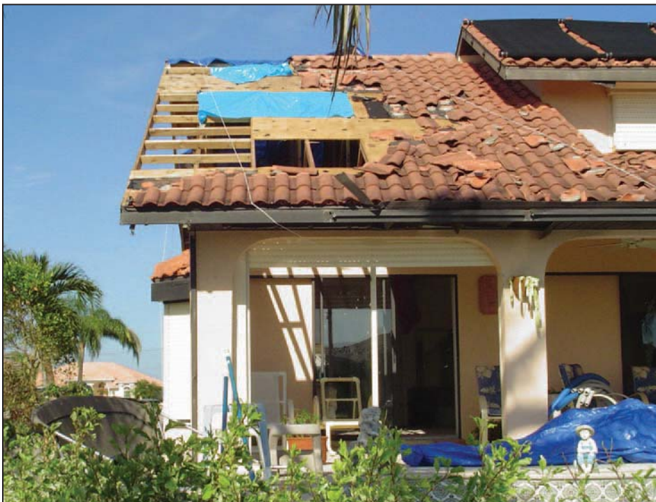
Figure 9-4. Load path failure in connections between roof decking and roof framing, Hurricane Charley (Punta Gorda, FL, 2004)
