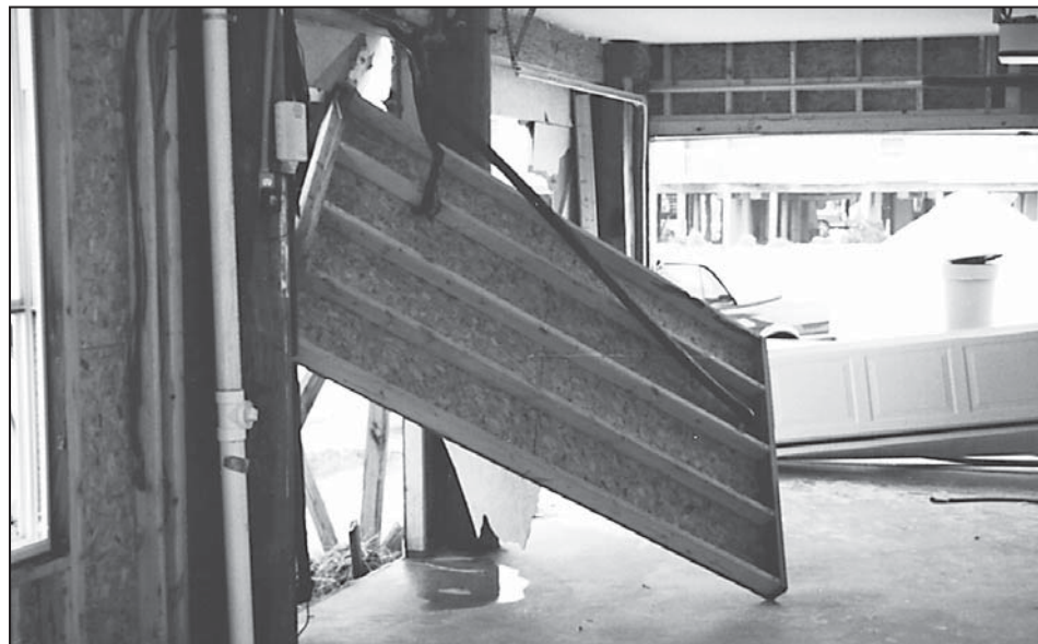
Figure 9-29. Breakaway wall panel prevented from breaking away cleanly by utility penetrations, Hurricane Opal (Florida, 1995)
