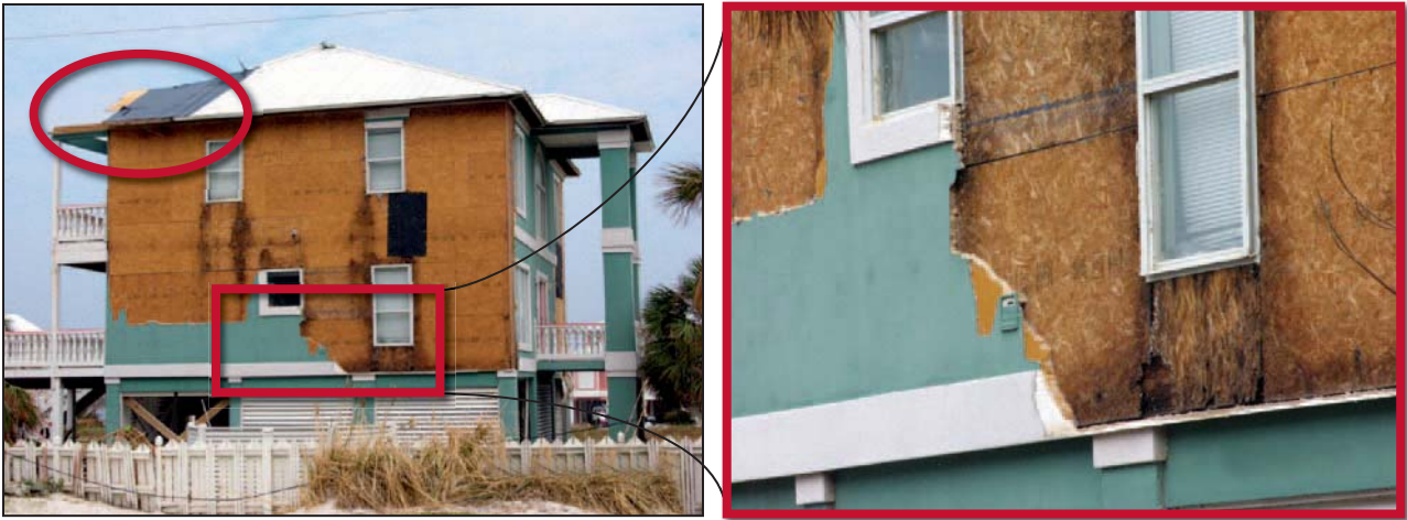
Figure 11-21. EIFS with a barrier design: blown-off roof decking (top circle); severely rotted OSB due to leakage at windows (inset). Hurricane Ivan (2004)
