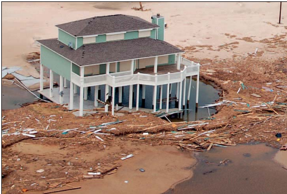
Figure 8-15. Deep scour around foundation piles, Hurricane Ike (Bolivar Peninsula, TX, 2008)
