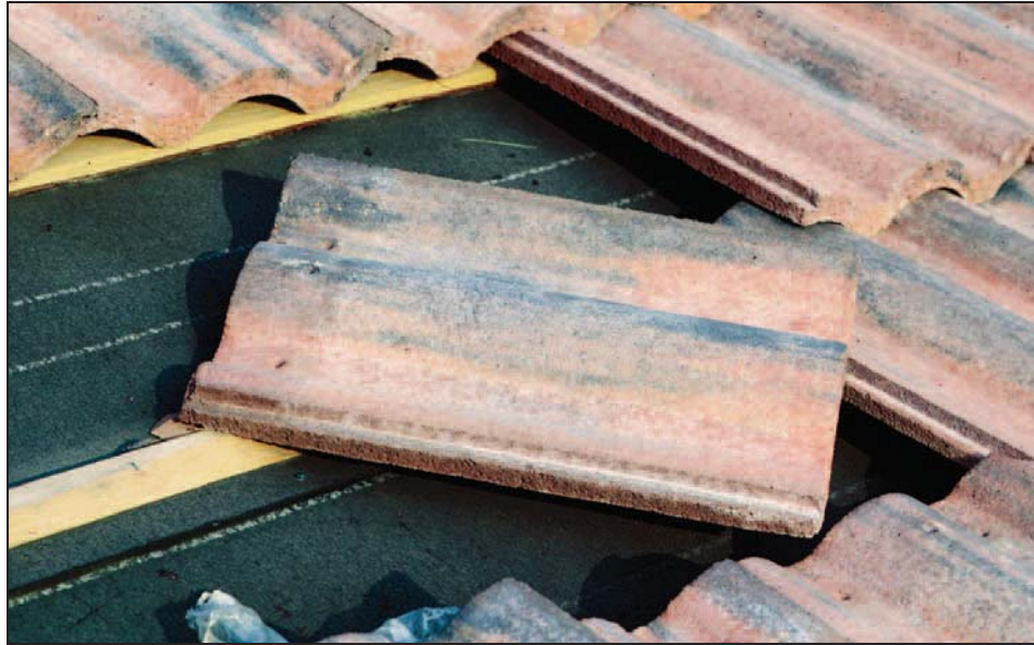
Figure 11-49. Area of the roof where tiles were not nailed to batten strips. Northridge Earthquake (California, 1994)
