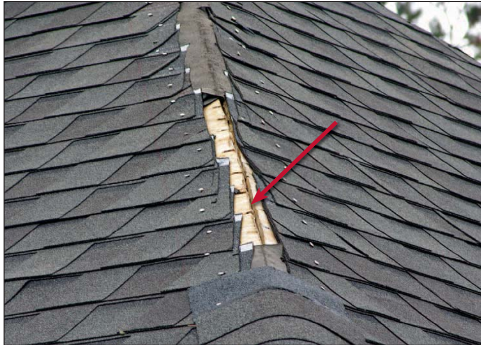
Figure 11-29. Underlayment that was not lapped over the hip; water entry possible at the sheathing joint (arrow). Estimated wind speed: 130 mph. Hurricane Katrina (Mississippi, 2005)
