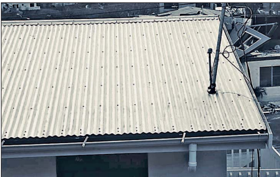
Figure 12-6. Damage caused by dropped overhead service, Hurricane Marilyn (U.S. Virgin Islands, 1995)
