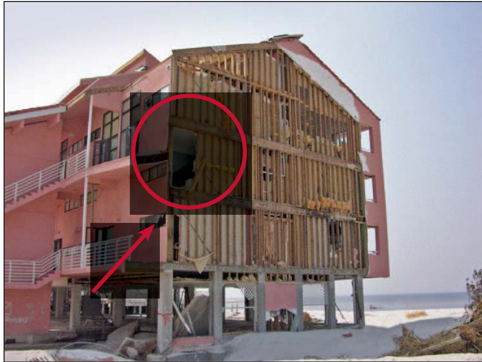
Figure 11-19. Blown-off EIFS, resulting in extensive interior water damage; detachment of the gypsum board or stud blow off (circle); two windows broken by debris (arrow). Estimated wind speed: 105 to 115 mph. Hurricane Ivan (Florida, 2004)
