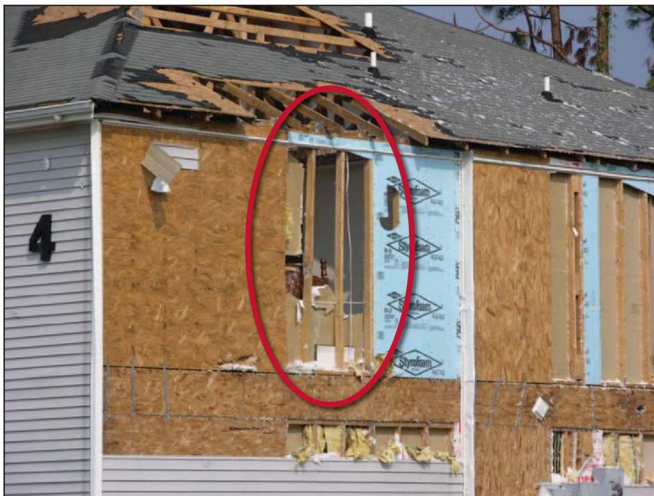
Figure 11-15. Blown-off vinyl siding and foam sheathing; some blow-off of interior gypsum board (circle). Estimated wind speed: 130 mph. Hurricane Katrina (Mississippi, 2006)
