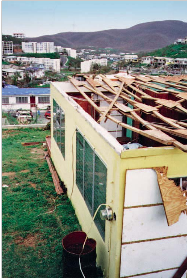
Figure 9-26. Gable-end failure caused by high winds, Hurricane Marilyn (U.S. Virgin Islands, 1995)
