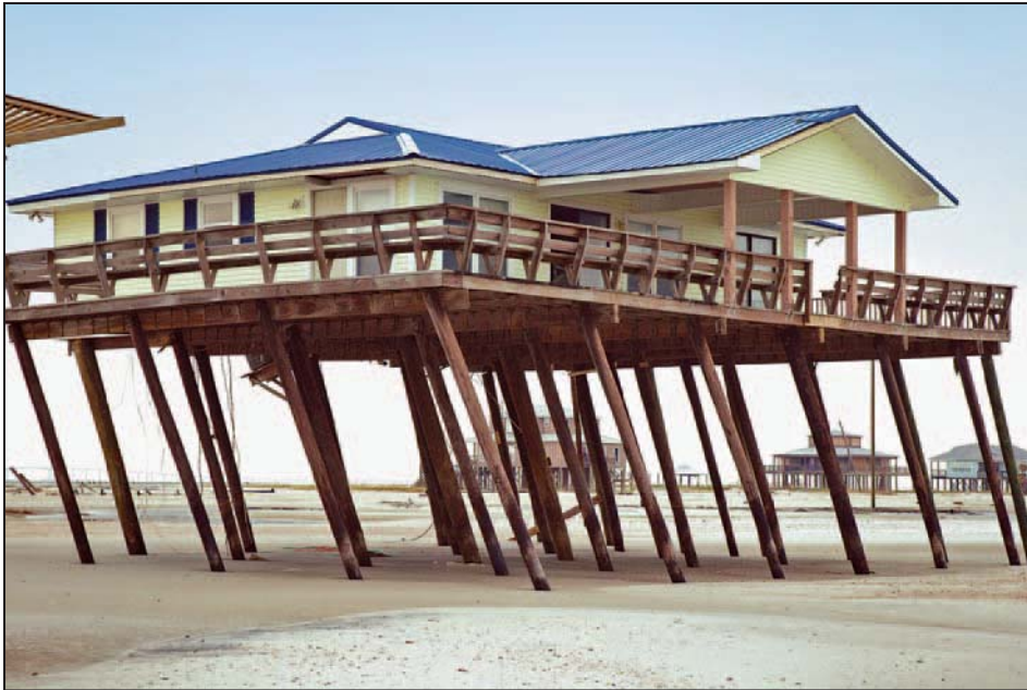
Figure 10-2. Near collapse due to insufficient pile embedment, Hurricane Katrina (Dauphin Island, AL, 2005)
