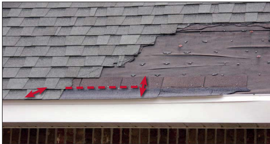
Figure 11-32. Incorrect installation of the starter course (incorrectly rotated starter, right arrow, resulted in self-seal adhesive not near the eave, dashed line). Estimated wind speed: 130 mph. Hurricane Katrina (Mississippi, 2005)
