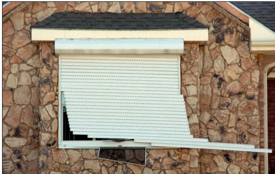
Figure 11-12. Roll-up shutter slats that detached from the tracks. The lack of a label makes it unclear whether the shutter was tested in accordance with a recognized method. Estimated wind speed: 110 mph. Hurricane Katrina (Louisiana, 2005)
