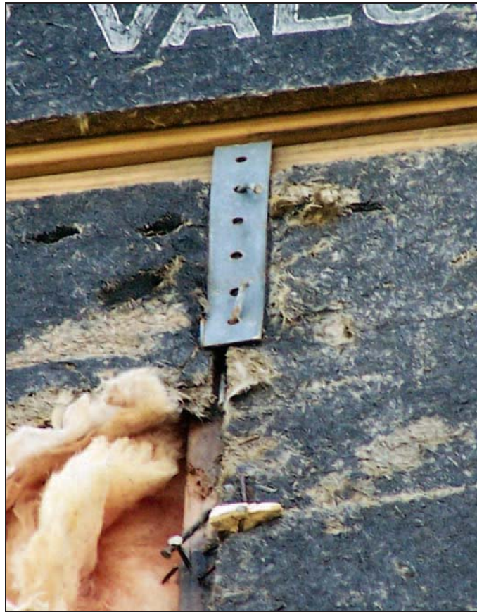
Figure 13-15. Connector failure caused by insufficient nailing
