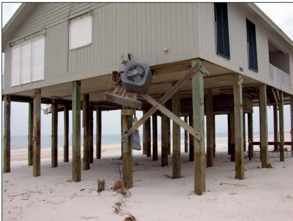
Figure 12-3. Small piles supporting a platform broken by floodborne debris
