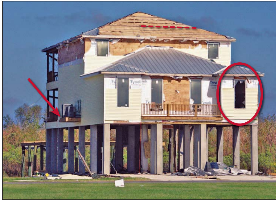
Figure 11-52. Blow-off of one of the nailers (dashed line on roof) caused panels to progressively fail; cantilevered condenser platform (arrow); broken window (circle). Estimated wind speed: 130 mph. Hurricane Katrina (Louisiana, 2005)
