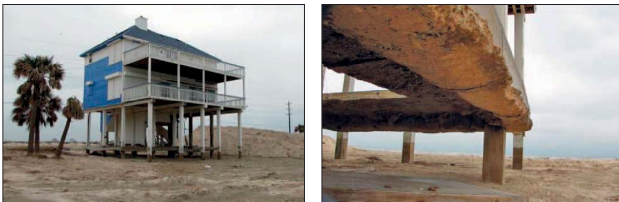
Figure 10-8. Scour around grade beam, Hurricane Ike (Galveston Island, TX, 2008)
