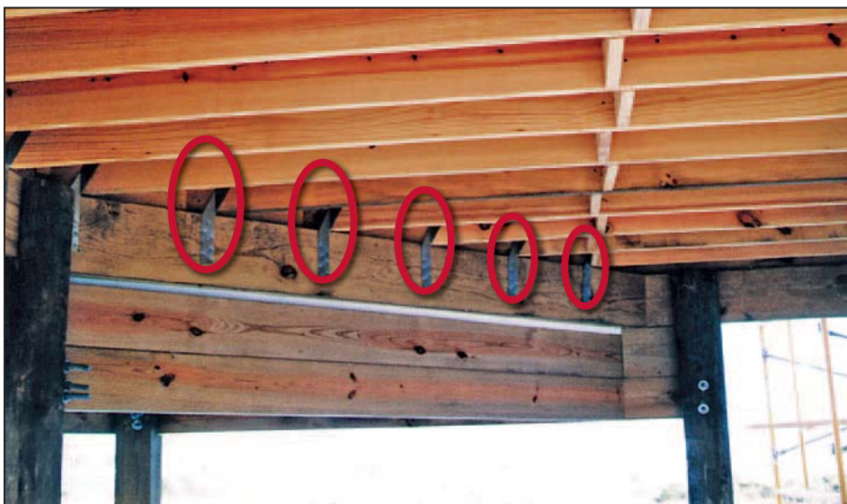
Figure 13-19. Proper use of metal twist strap ties (circled); solid blocking between floor joists
