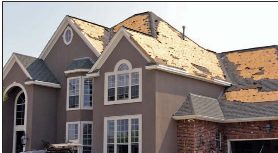
Figure 11-25. Typical underlayment attachment; underlayment blow-off is common if the shingles are blown off, as shown. Estimated wind speed: 115 mph. Hurricane Katrina (Louisiana, 2005)
