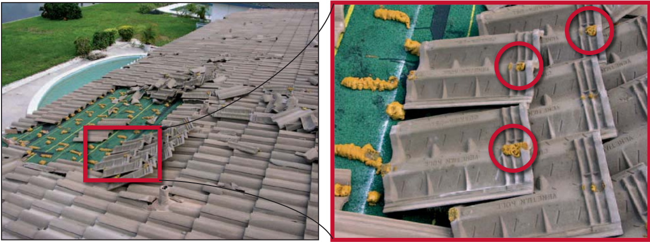
Figure 11-43. Blown-off adhesive-set tile. Note the very small contact area of the foam at the tile heads (left side of the tiles) and very small contact at the nose (circles). Estimated wind speed: 140 to 160 mph. Hurricane Charley (Florida, 2004)
