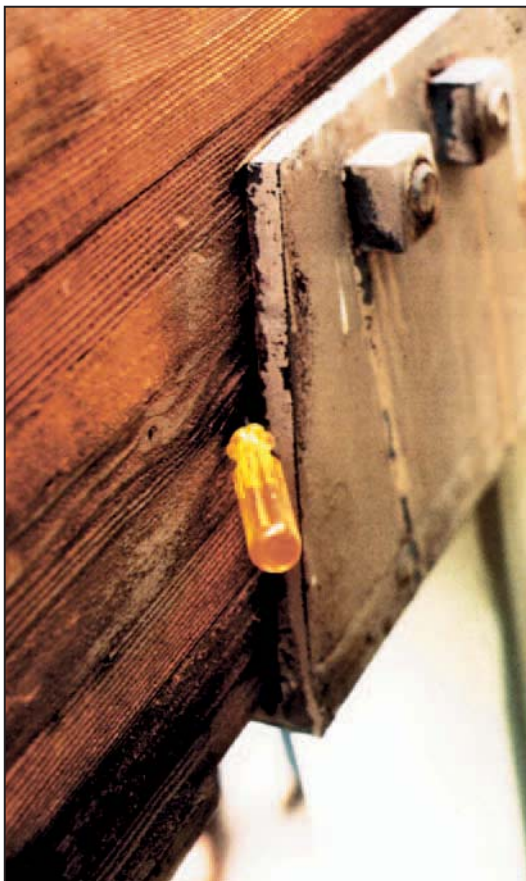
Figure 14-2. Wood decay behind a metal beam connector
