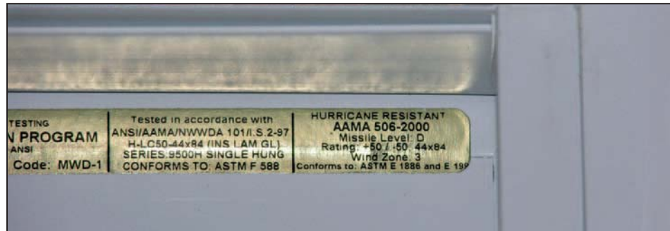
Figure 11-11. Design pressure and impact-resistance information in a permanent window label. Hurricane Ike (Texas, 2008)
