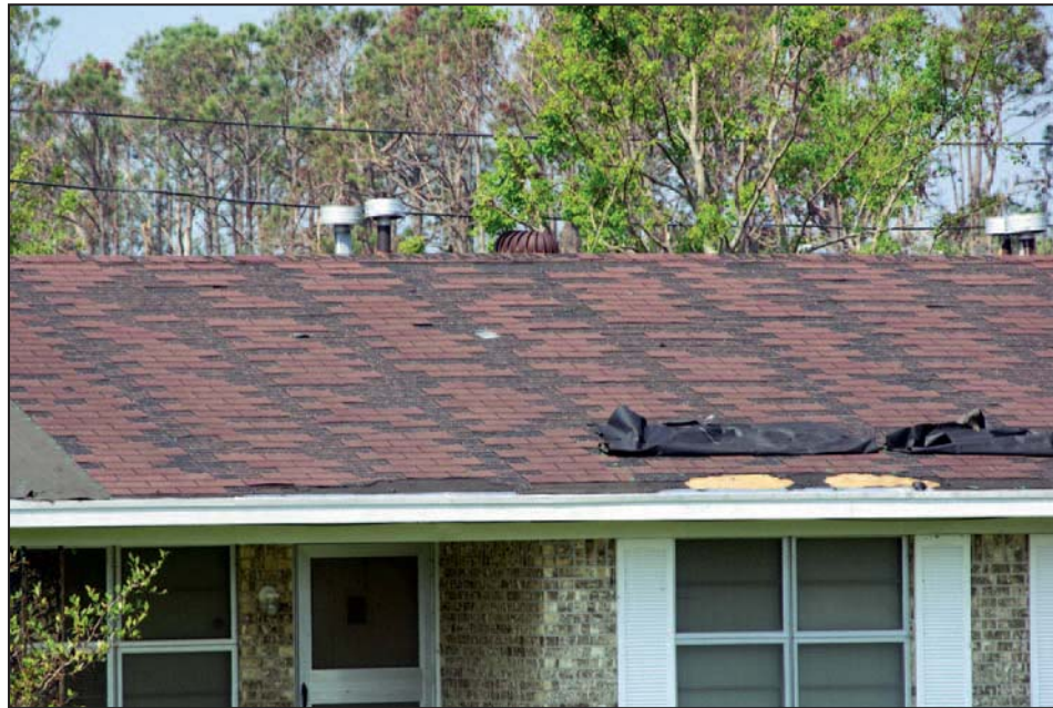
Figure 11-38. Shingles that unzipped at the band lines because the raking method was used to install them. Estimated wind speed: 135 mph. Hurricane Katrina (Mississippi, 2005)
