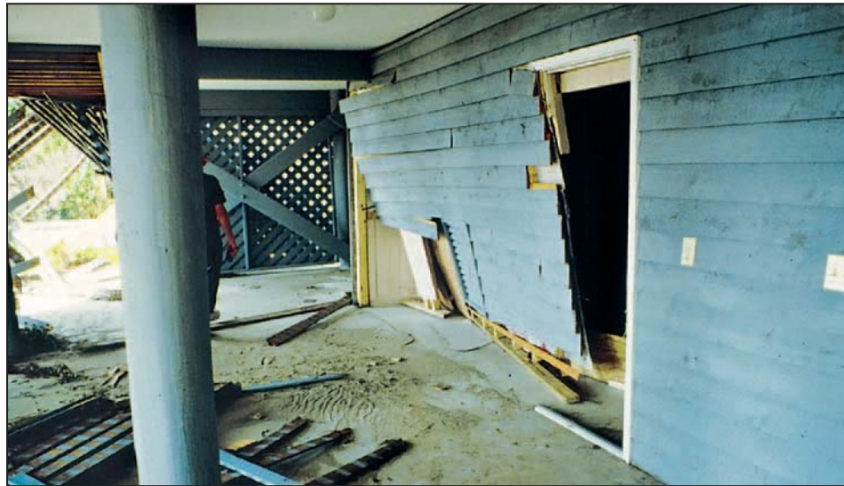
Figure 9-28. Typical failure mode of breakaway wall beneath an elevated building—failure of the connection between the bottom plate of the wall and the floor of the enclosed area, Hurricane Hugo (South Carolina, 1989)
