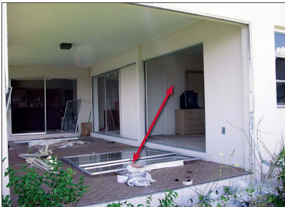
Figure 11-5. Sliding glass doors pulled out of their tracks by wind suction. Estimated wind speed: 140 to 160 mph. Hurricane Charley (Florida, 2004)
