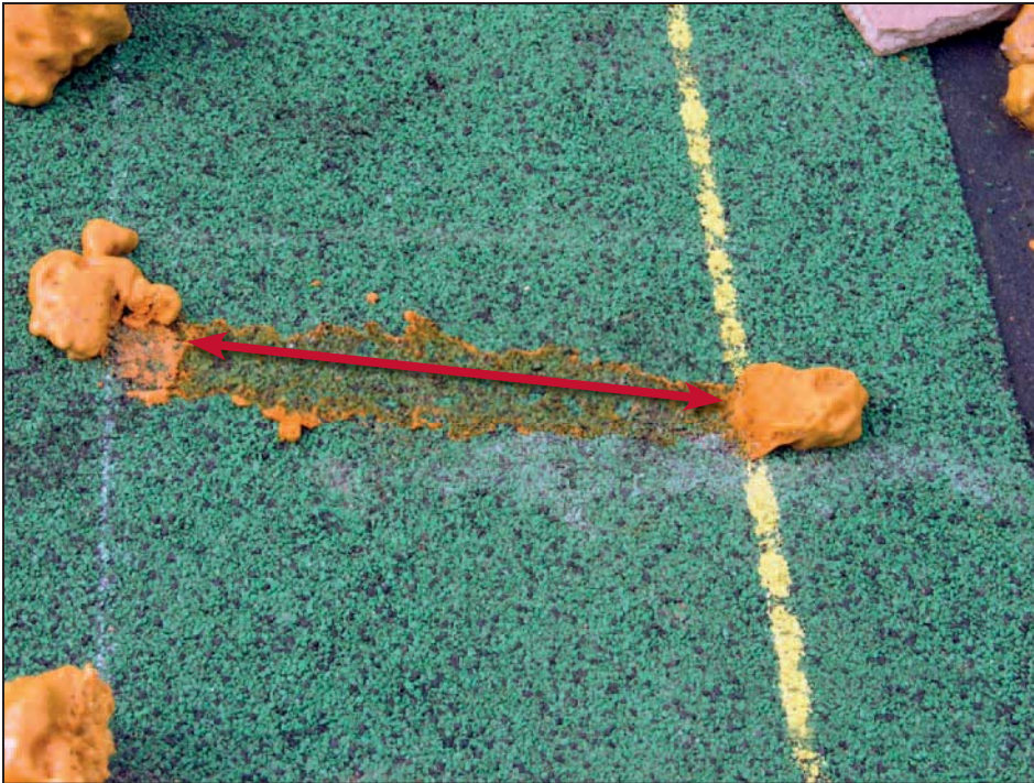
Figure 11-44. Adhesive that debonded from the cap sheet
