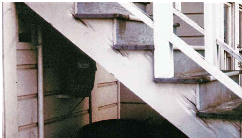
Figure 13-13. Deterioration in a notched stair stringer
