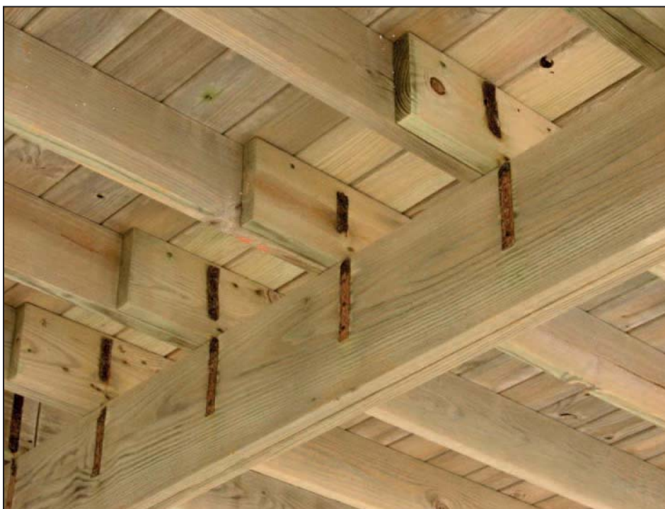
Figure 14-3. Severely corroded deck connectors
