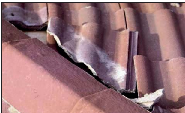
Figure 11-51. Tile that slipped out from under the hip tiles. Northridge Earthquake (California, 1994)
