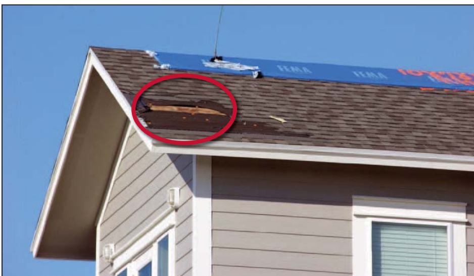
Figure 11-31. Loss of shingles and underlayment along the rake. Estimated wind speed: 110 mph. Hurricane Ike (Texas, 2008)
