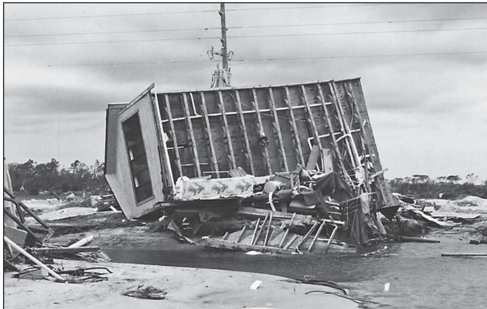
Figure 9-2. Load path failure in connection between home and its foundation, Hurricane Fran (North Carolina, 1996)
