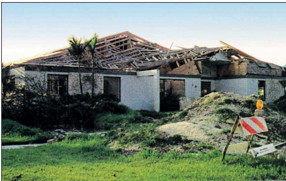
Figure 9-21. Gable-end failure, Hurricane Andrew (Dade County, FL, 1992)
