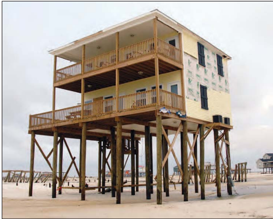
Figure 2-14. Successful example of well-elevated and embedded pile foundation tested by Hurricane Katrina. Note adjacent building failures (Dauphin Island, AL, 2005)
