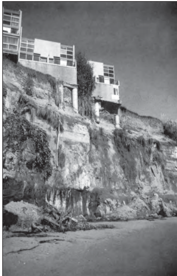
Figure 3-37. Bluff failure by a combination of marine, terrestrial, and seismic processes led to progressive undercutting of blufftop apartments at Capitola, CA, where six of the units were demolished after the 1989 Loma Prieta earthquake SOURCE: GRIGGS 1994, JOURNAL OF COASTAL RESEARCH , USED WITH PERMISSION
