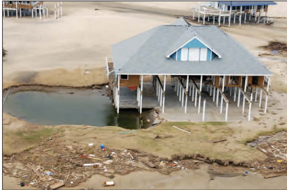
Figure 3-49. Residential foundation that suffered severe scour on Bolivar Peninsula, TX (Hurricane Ike, 2008)
