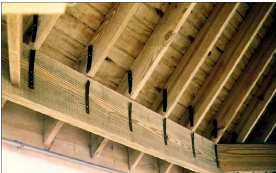
Figure 3-17. Example of corrosion, and resulting failure, of metal connectors
