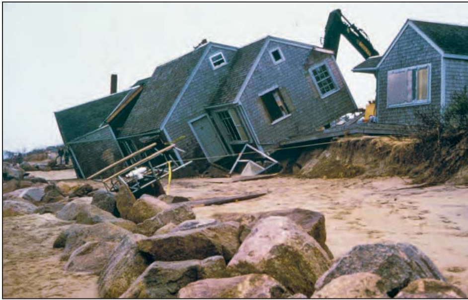
Figure 3-36. Undermined house at Chatham, MA, in 1988; nine houses were lost as a result of the formation of the new tidal inlet shown in Figure 3-35 SOURCE: JIM O'CONNELL, USED WITH PERMISSION
