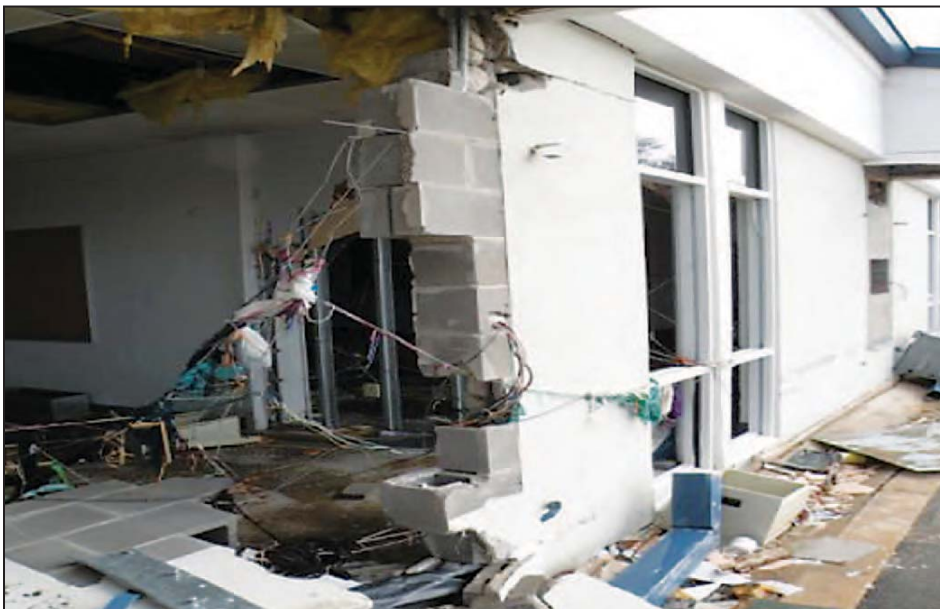
Figure 2-10. School located approximately 1.3 miles from the Gulf shoreline damaged by storm surge and small waves, Hurricane Ike (Cameron Parish, LA, 2008)
