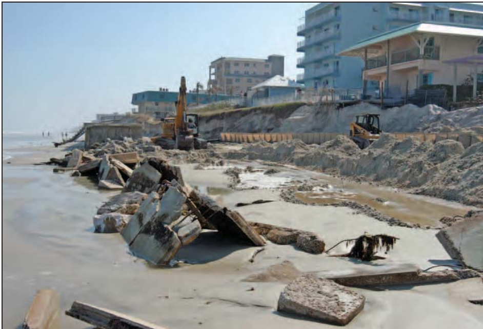
Figure 3-32. Erosion and seawall damage in New Smyrna Beach, FL, following Hurricane Jeanne in 2007
