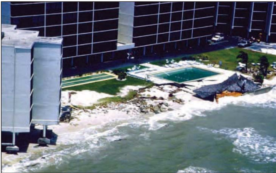
Figure 4-24. Beach erosion and damage due to a destroyed bulkhead at Bonita Beach, FL, from a subtropical storm
