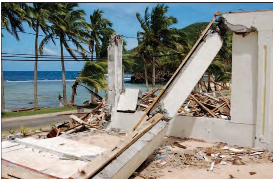
Figure 3-12. Damage from the 2009 tsunami (Amanave, American Samoa)
