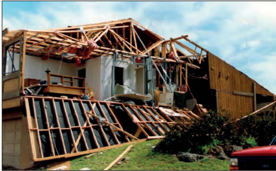
Figure 3-8. End-wall failure of typical first-floor masonry/ second-floor wood-frame building in Dade County, FL (Hurricane Andrew, 1992)
