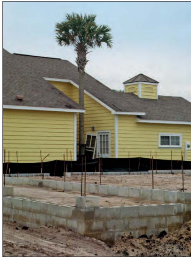
Figure 4-25. (below) Notching the building and roofline around a tree can lead to roof and envelope damage during a high-wind event
